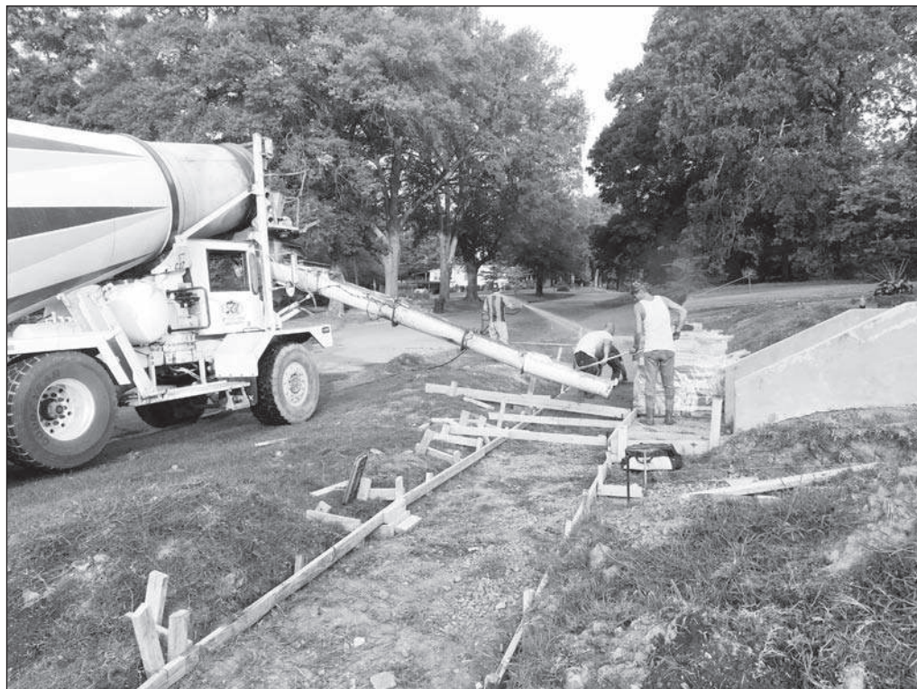
EARLY MORNING WORK. Workmen pour and smooth a sidewalk at the E.A. Williams Chapel and Museum, early Tuesday morning. The crews were due to return Wednesday to pour another sidewalk connecting to the handicapped entrance to the museum.
