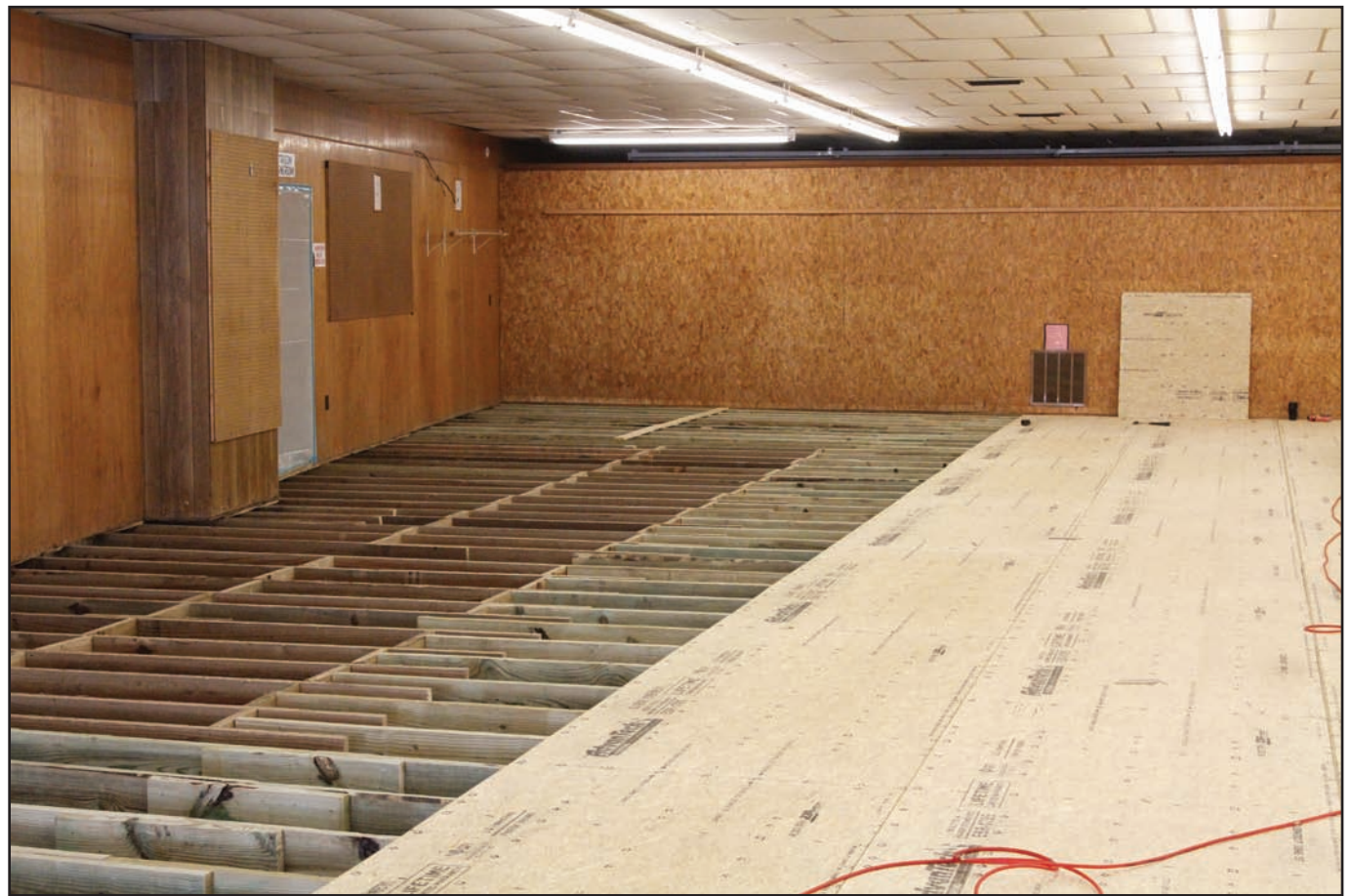
DEWAYNE HOLLOWAY | Montgomery County News Work continues on the floor renovations at the Montgomery County Nursing Home Ladies Auxiliary Thrift Store in Mount Ida.
