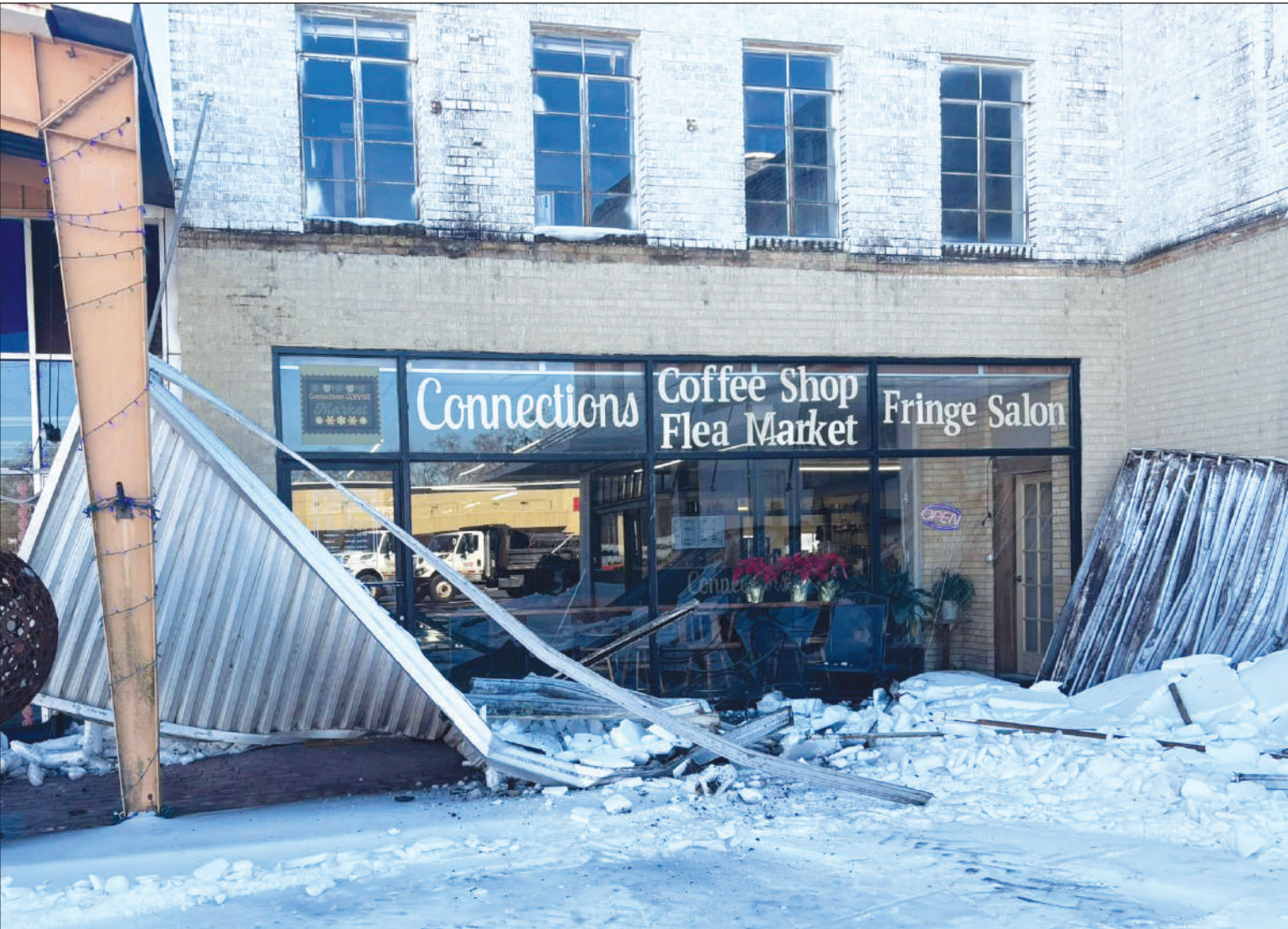
BUSINESS INTERRUPTION ... Connections Coffee on the Pike County Courthouse square was closed last Friday after the weight of ice forced the awning above the store to collapse. Store owners noted on social media that they were grateful that no one was injured in the accident.
